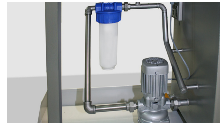
Pump and filter
